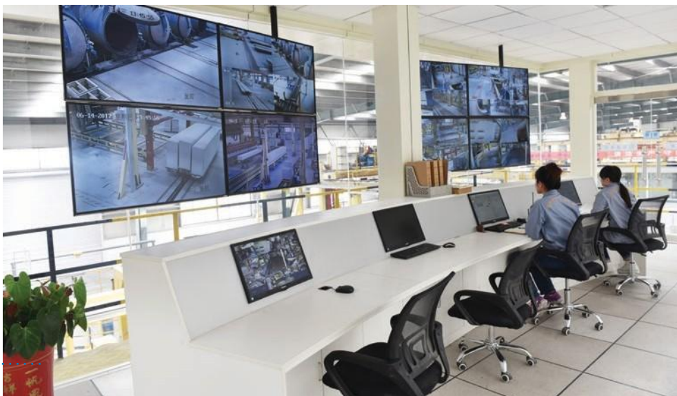
Fig. 8: Central control room.
